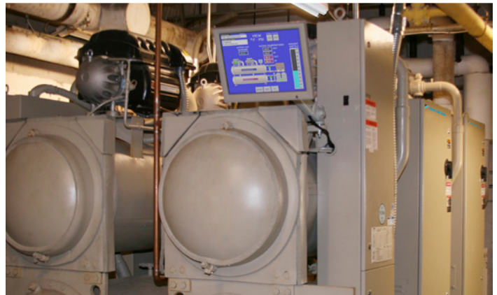
The Daikin Magnitude chillers at One Crawford were commissioned in June 2007.
