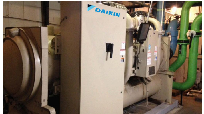
Reduced kilowatt usage of the high-efficiency Magnitude chiller contributes to the owner's energy savings.
