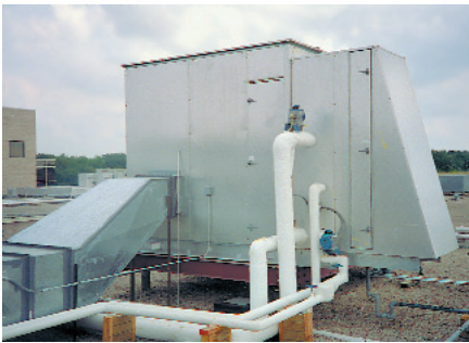
Because the MDAire system was installed on the roof and connected at the fresh air inlet, it was easy to retrofit and upgrade the old HVAC system without interrupting normal hospital operations
