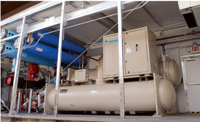
Specifically designed for mission-critical facilities, each of the Daikin modular plants at Phoenix NAP includes multiple internal redundancies.
